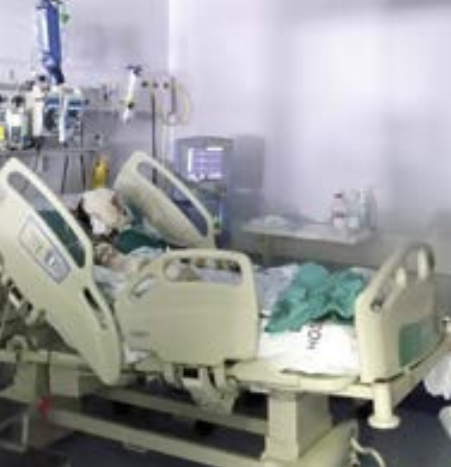
Photo 1: Illustration of non-functional UVGI fixtures in an ICU ward at a regional hospital in South Africa.
