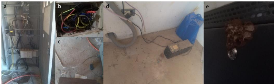
Fig. 1. The conditions of the electrical panels, wiring and equipment.
