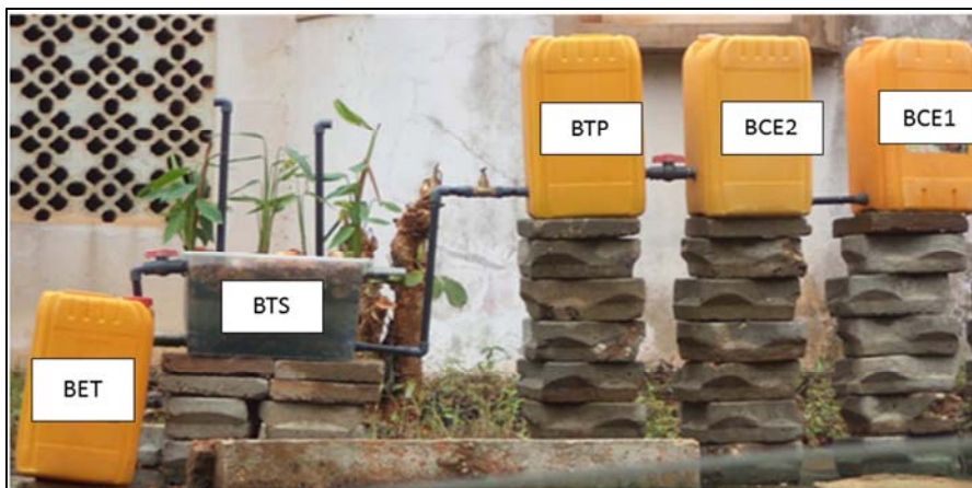
Figure 3. Autonomous Gray Water Treatment System (SAUTEG).
